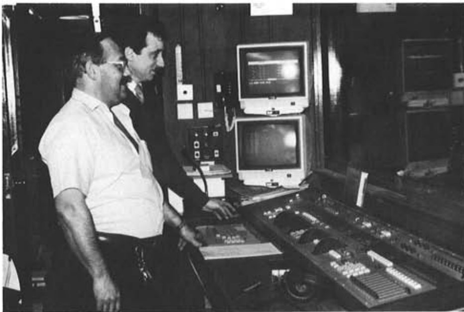
Andy Kent, the Theatre Royal's chief electrician, pictured with Northern Light's Jonathan Allen in the FOH lighting control room. The board is a Strand Galaxy 2 Premier.
